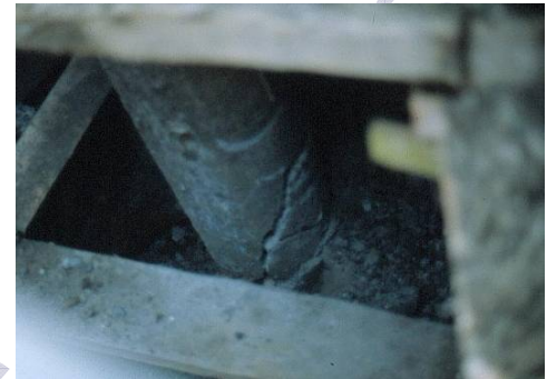
Crack detected at 3.5m using TDR
