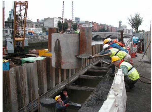
Fig 3. Four tonne, concrete mass sliding on a central reinforcing bar. Foundations for Bridge over the River Liffey, Blackhall Place, Dublin.
